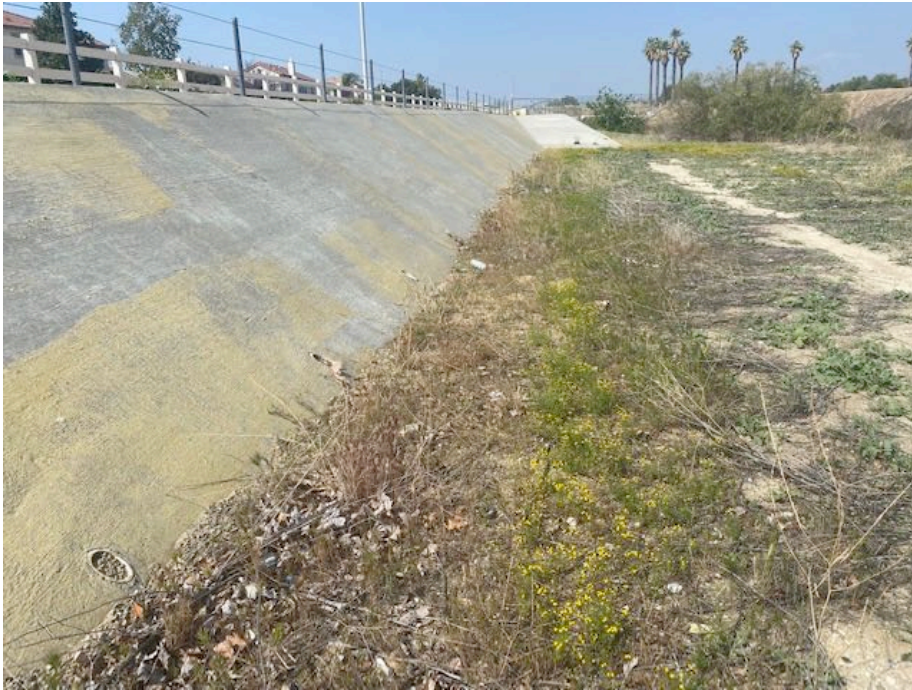
Photograph 31: Weep holes at the base of a concrete flood control wall on the west side of the channel.
